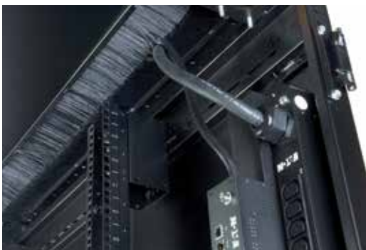
RP Series rack with 2 installed Eaton ePDUs
